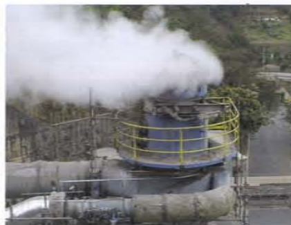
Figure 2. Stack before dedusting
