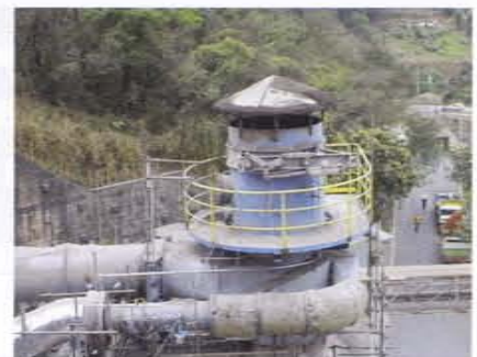
Figure 3. Stack with dedusting device in operation
